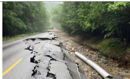
Heavy rains damage roads
