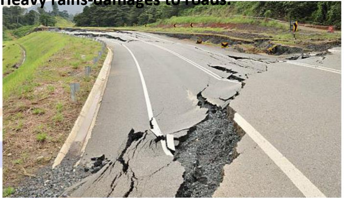
Heavy rains-damages to roads.
